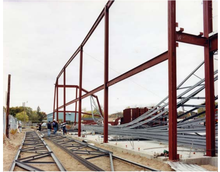
Figure 6 View of collapse looking in a northeast direction from a point near Column A-53.
