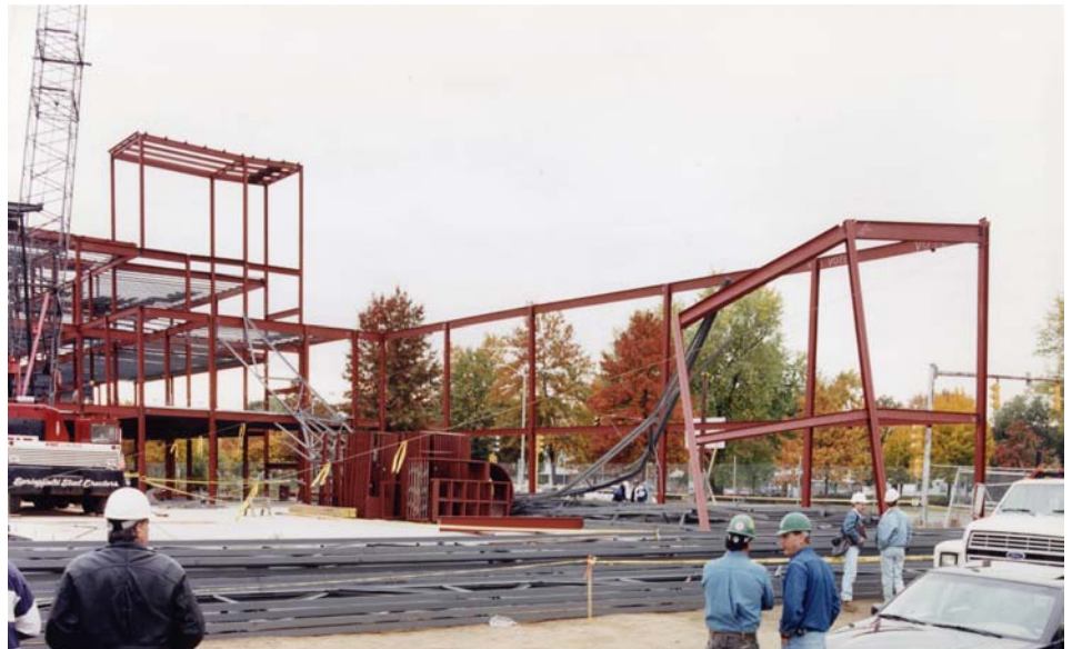
Figure 1 View of collapse taken the same day, looking southwest.
