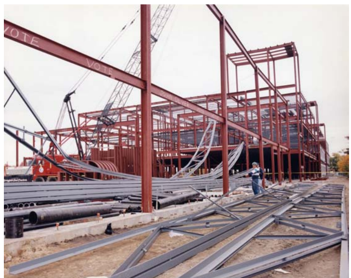
Figure 7 View of collapse looking southeast. Framing running from left foreground to the right background is Line A.
