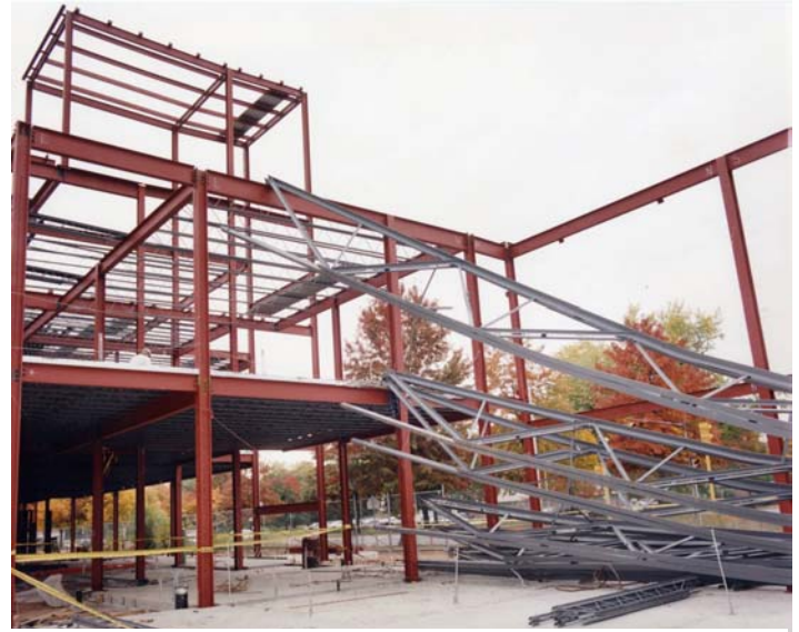
Figure 8 South end of collapsed joists. The Line 53 steel runs from the left to the right; The Line A steel is on the right. LS-1 is hung up on the roof girder; LS-2 and LS-3 are hung up on the 2nd floor of the classroom building.
