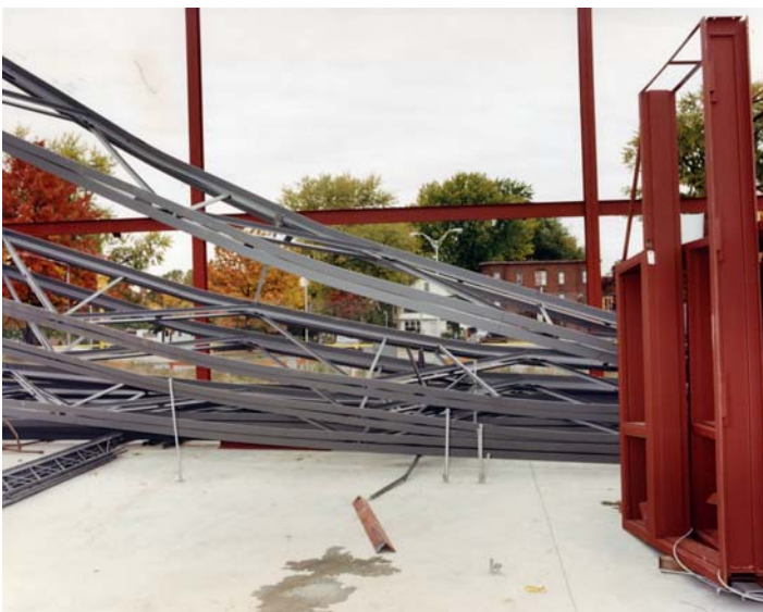
Figure 9 View of joists to the right of that shown in Figure 8. The angle on the ground is one of the strong backs.
