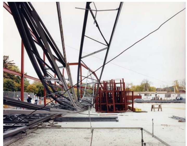
Figure 10 View under joists looking north. LS-1 is hung up in the air on the right. The near ends of LS-2 and LS-3 were also hung up in the air.
