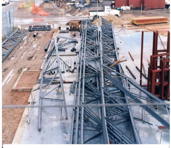
Figure 11 View of collapse from 2nd floor of classroom building, looking north, after the joists that were hung up on the framing were cut down, and after the framing on Line A and Line 65 was dismantled. The north half of LS-1 is on the left; the south half of LS-1 is lying across the right pile.
