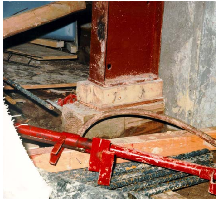
Figure 7. Wood blocking supporting base plate of temporary steel column on Line 5; believed to be at the most northerly end of the formwork that collapsed. (The column shown did not collapse).
