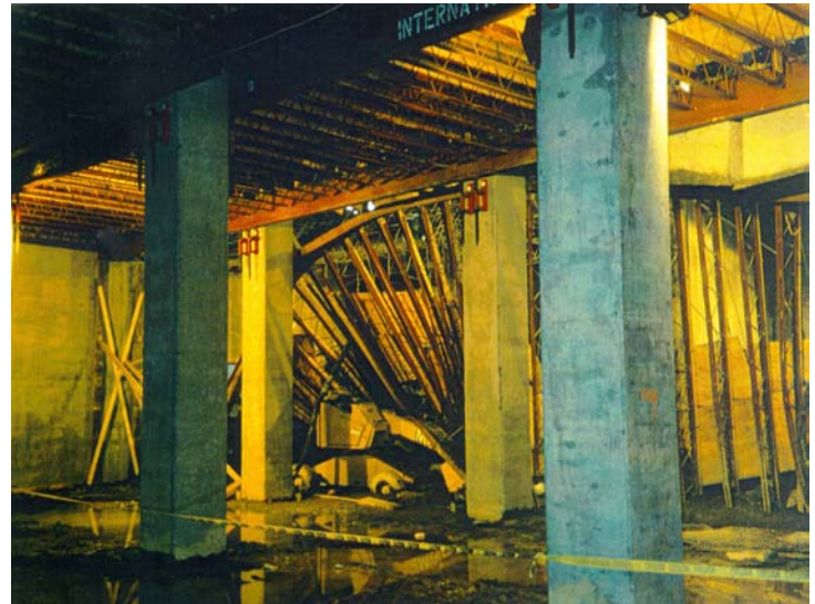
Figure 1. View of collapse from below. Photo taken from under flying formwork that did not collapse.
