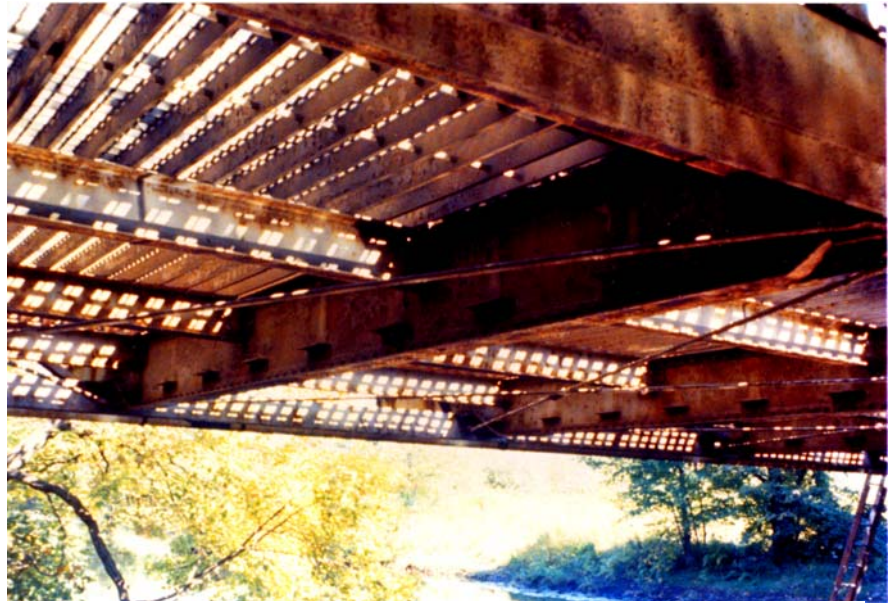
Figure 5. View of bottom of Main Street Bridge, circa 1978, showing seats on the floor beams for the original timber stringers.
