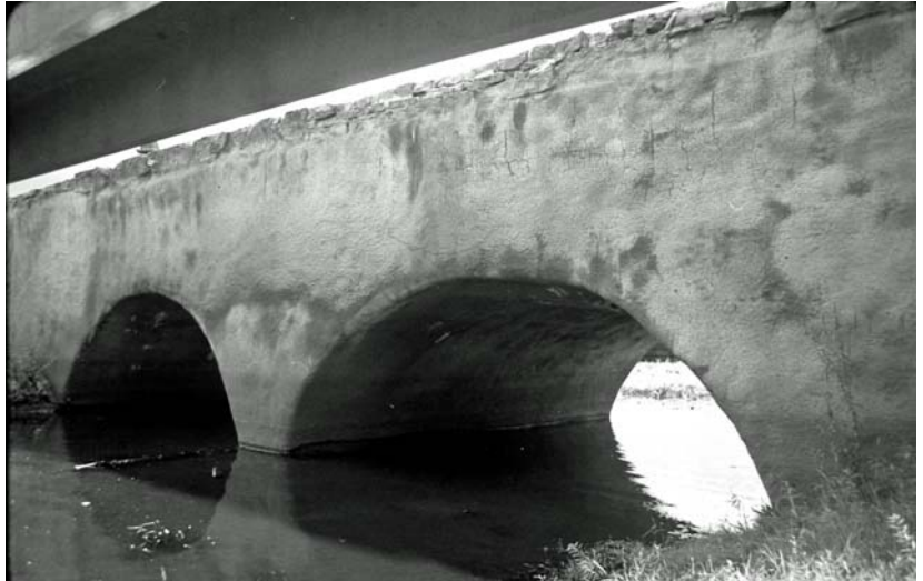
Figure 2. Downstream side of the Winter Street Bridge as it appeared in 1977. The bottom of the footbridge can be seen in the upper left foreground.
