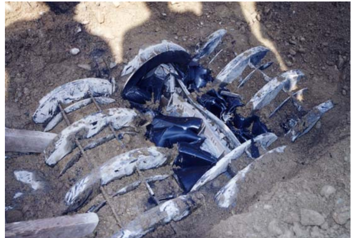
Figure 6. Test Pit No. 2 showing the top of a main chamber removed. The buckled legs of the main chamber are partially visible, and extend under the top arch fillers on each side.
