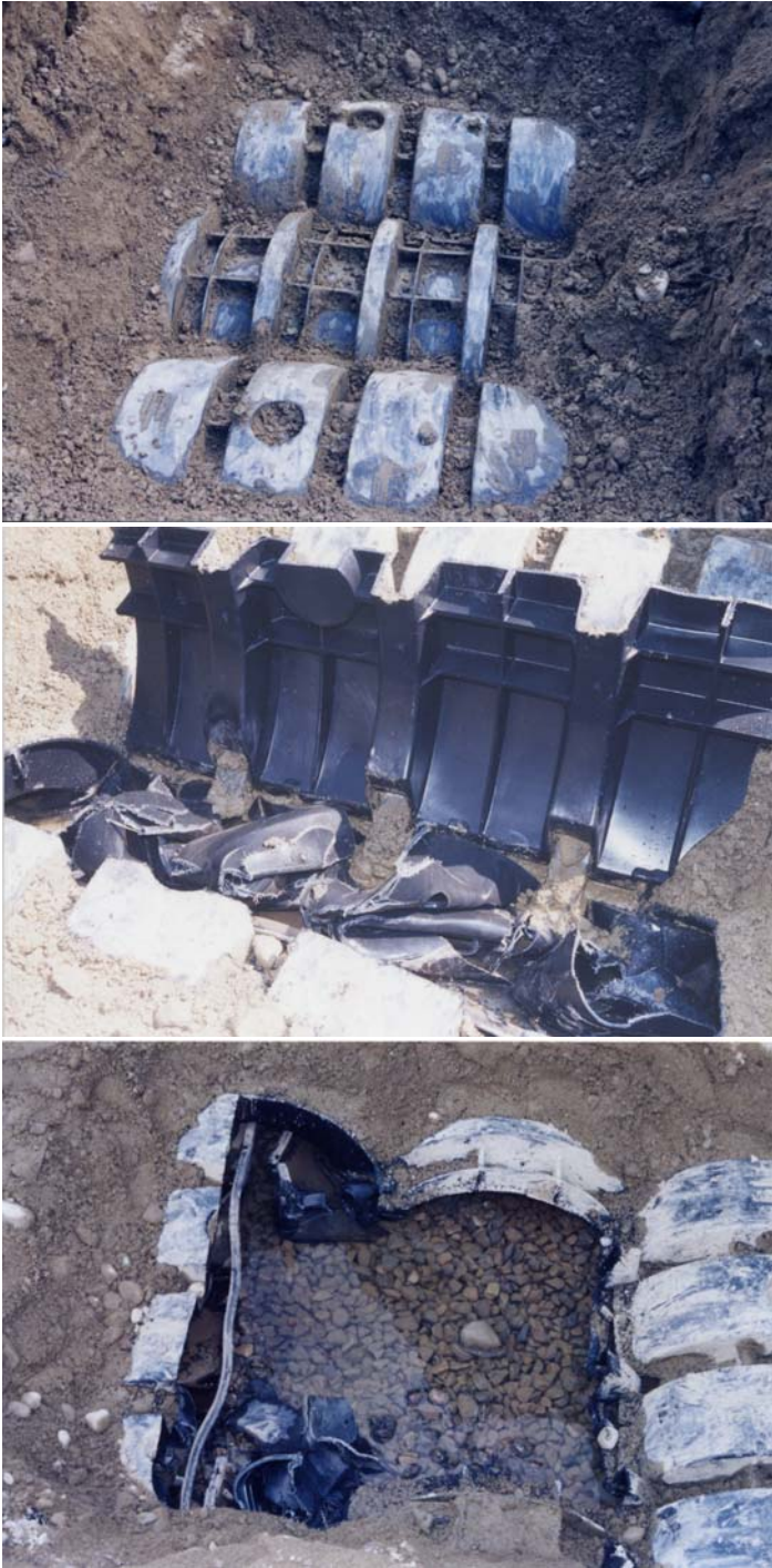
Figure 7. Test Pit No. 1. Top photo: center arch is top of a main chamber; adjacent arches are fillers over the spaces between main chambers. Center photo: near side arch filler cut away revealing collapsed legs of main chambers. Bottom photo: after removal of main chamber arch and near side arch filler. All arches are resting on the crushed stone base, 24" below their original positions.
