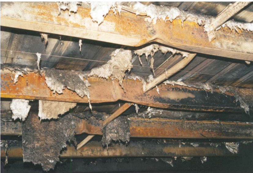
Figure 6. Twisted and kinked roof purlins. Insulation has been destroyed by the fire and the metal roofing is exposed.
