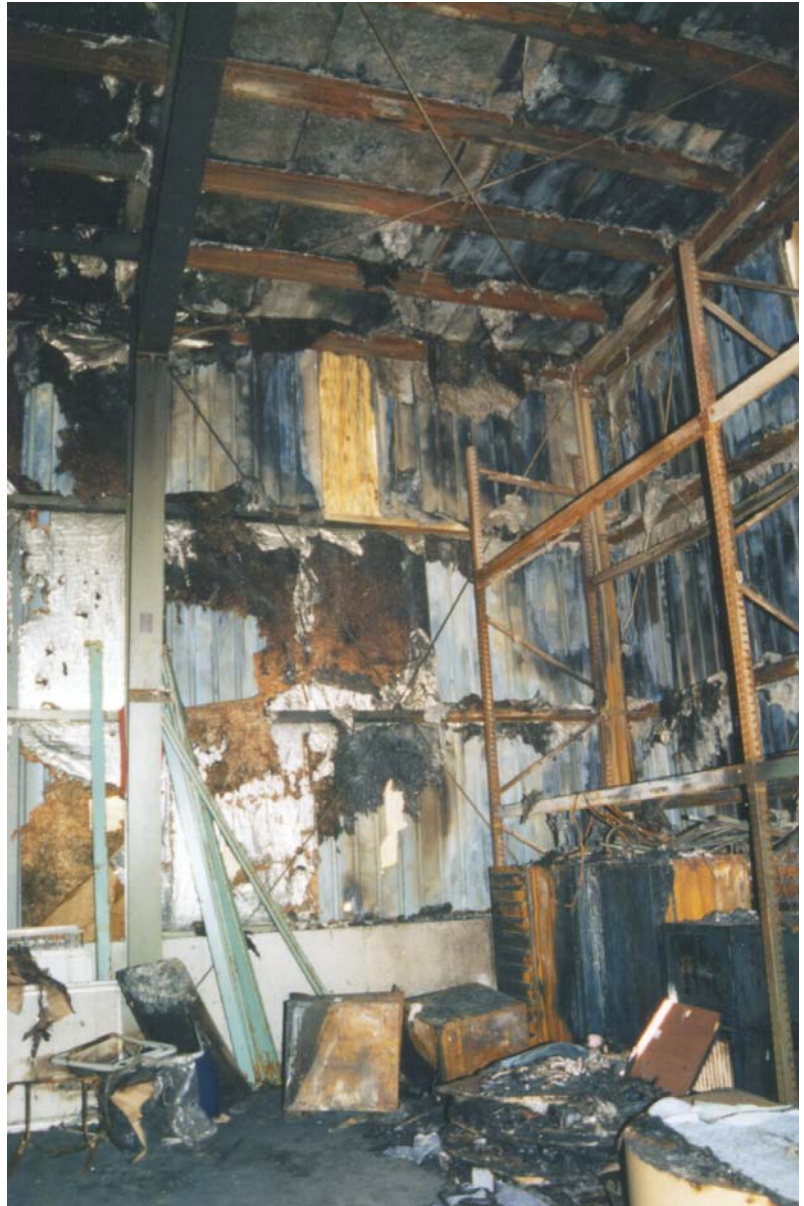
Figure 7. Fire damage at corner A-9. Corner column A-9 is twisted; the roof beam on Line 9, framing to this column, is twisted, and the roof purlins and wall girts near this corner are all twisted. Note the rod cross-bracing in the walls and at the bottom of the roof purlins; these are all loose as a result of the fire.
